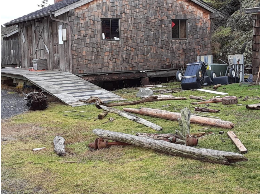
Debris left behind after January flooding
